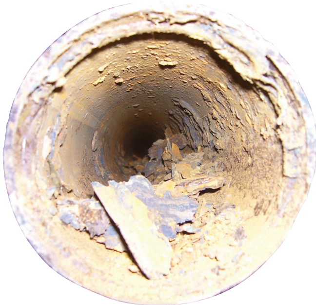
Internal Pipe Corrosion
